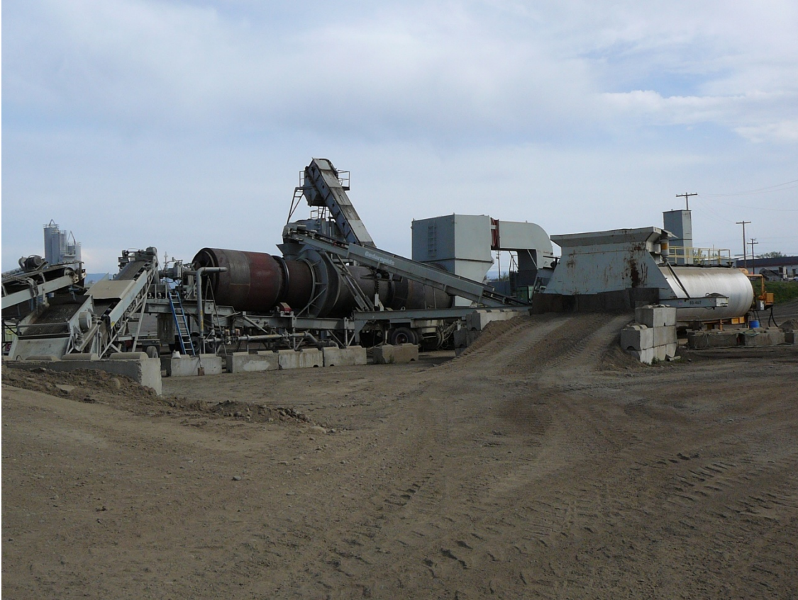
FIGURE 2 Granite Northwest — Walla Walla, WA Portable Asphalt Plant
