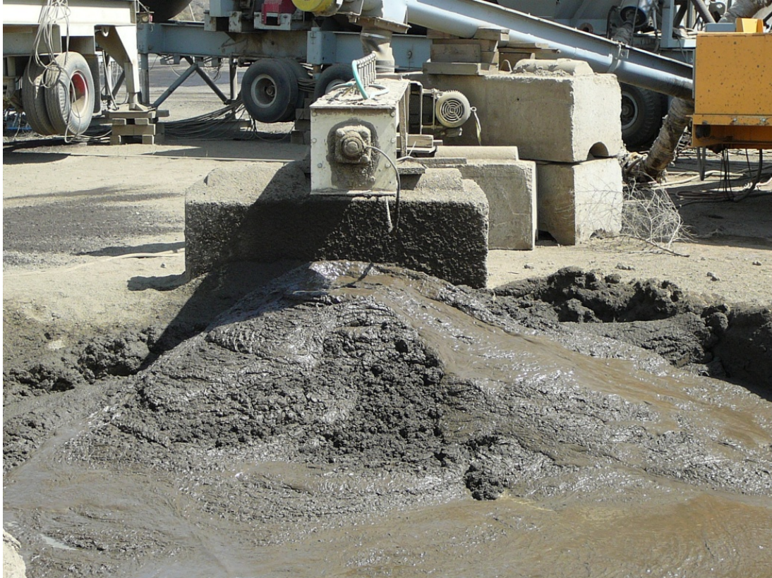
FIGURE 3 Waste Auger System for Baghouse, Showing Full Mixing of Water and Dust
