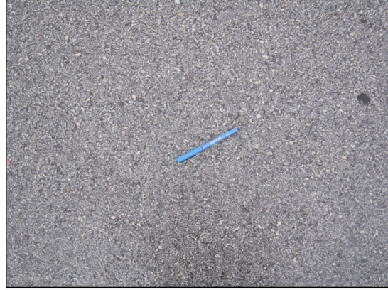
Figure 8: WMA 11/2010: Close up of pavement
