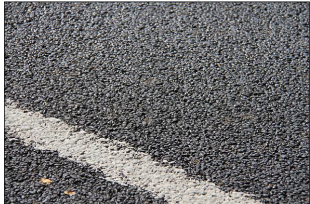
Figure 5.4: Gencor Ultrafoam 06/2010: Close-up view.
