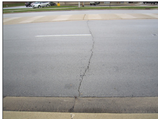
Figure 6: Control 11/2010: Transverse Crack
