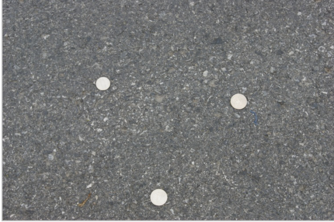
Figure 7: WMA May 3, 2011: Close up of pavement
