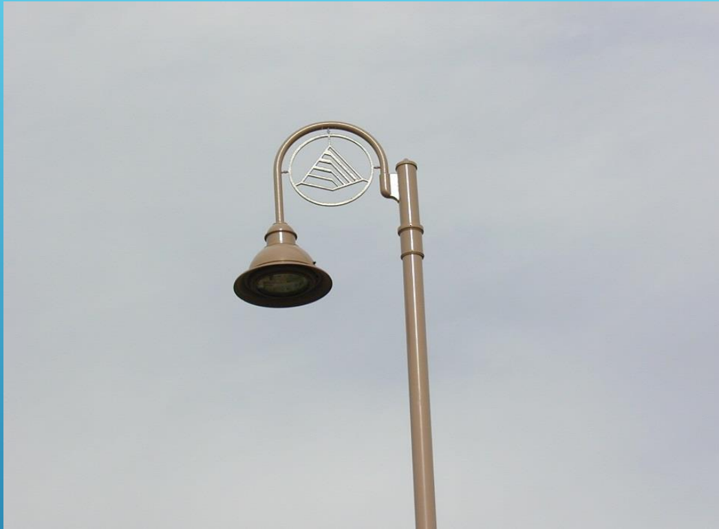
Street Lights-7,716 198 City Owned
