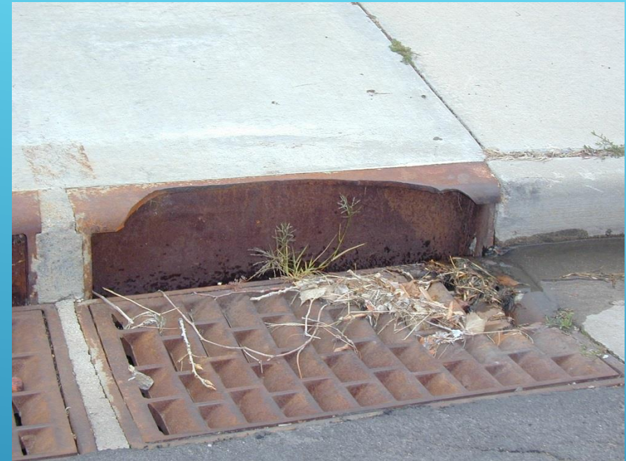
Storm Water System- 2,075 Inlets 183 Miles of Storm Sewer
