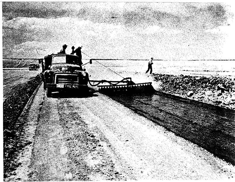
FIGURE VIII-3. Placing asphalt membrane lining, Rocky Mountain Arsenal, Colorado (U.S. Bureau of Reclamation).
