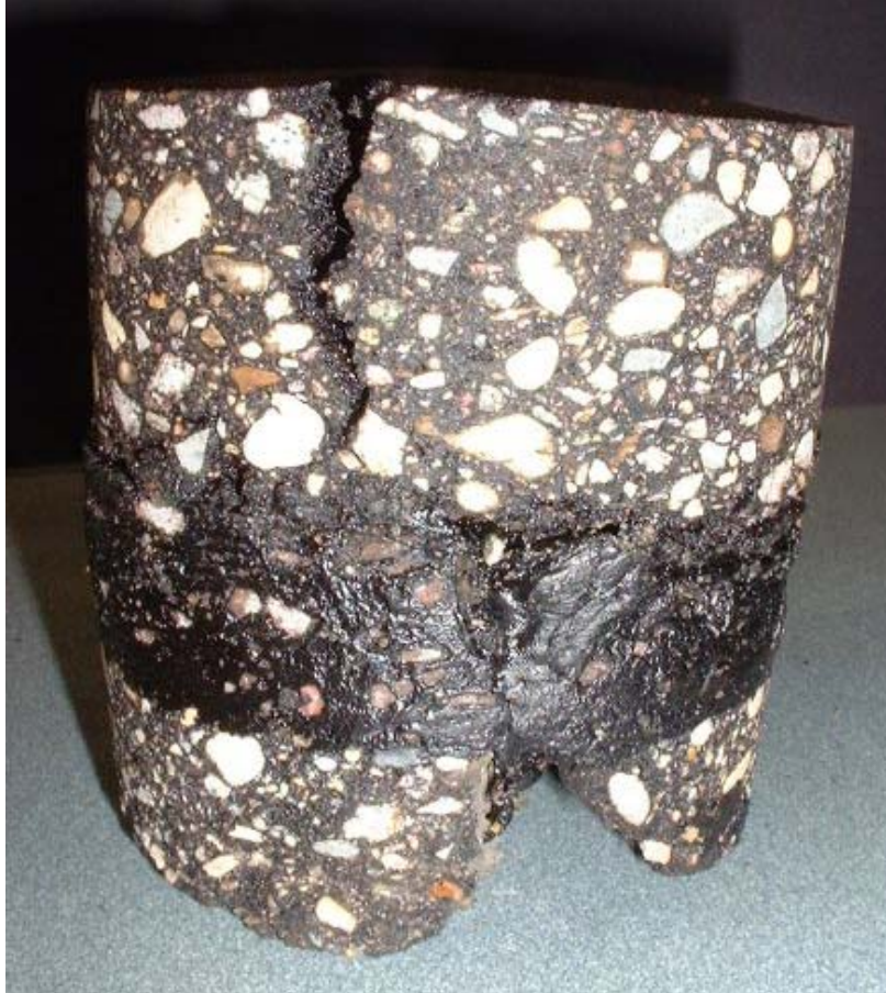
Figure 6.8. Core removed from pavement near milepost 34 on TH 22.
