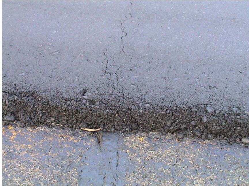
Figure 6.10. Bump at sealed crack on CSAH 9 in Lyon County.
