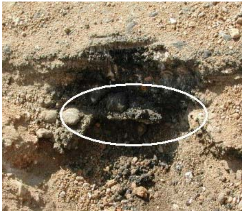
Figure 4.4. Cutaway section at pavement edge showing crack sealant at interface – Pipestone County.
