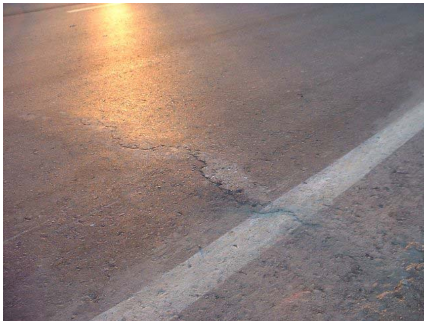
Figure 6.7. A Large bump near milepost 19 on TH 22 near Wells, Minn.
