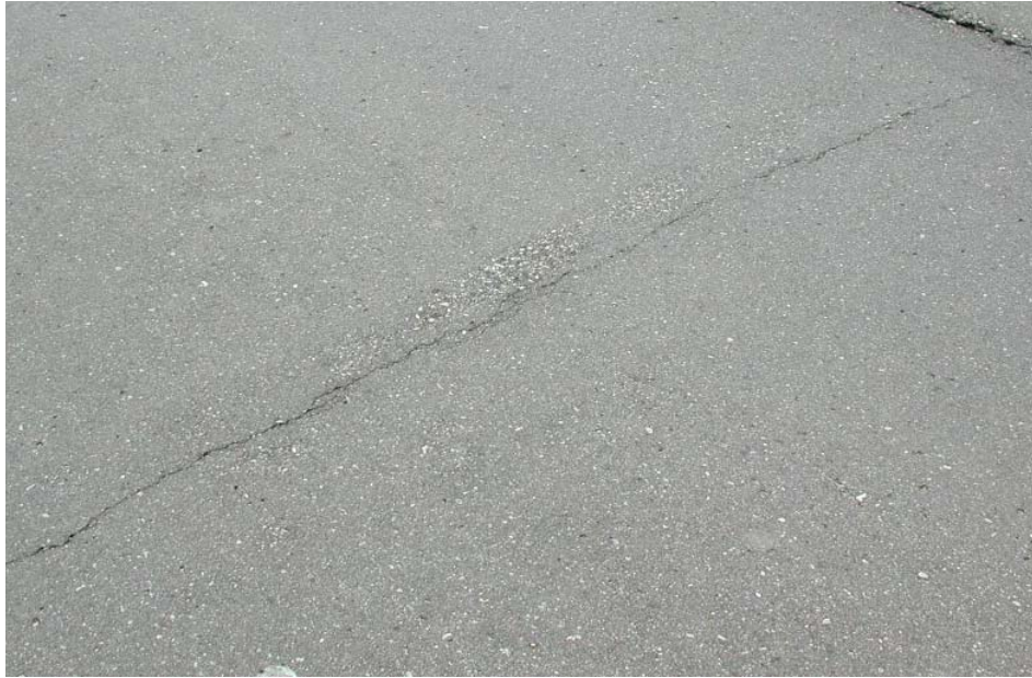
Figure 4.1. Transverse crack with overlay-related bump – Pipestone County.
