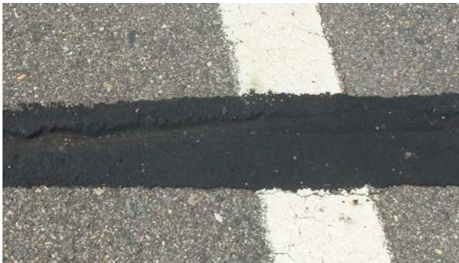
Figure 4.5. Routed and sealed crack, no overlay, Todd County.
