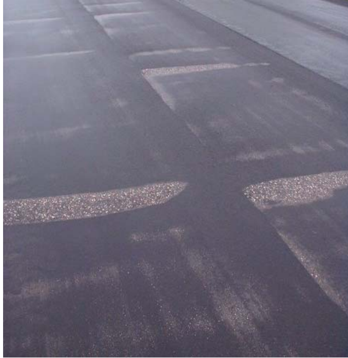
Figure 6.15. Bumps in 200-foot section in Cottonwood County.
