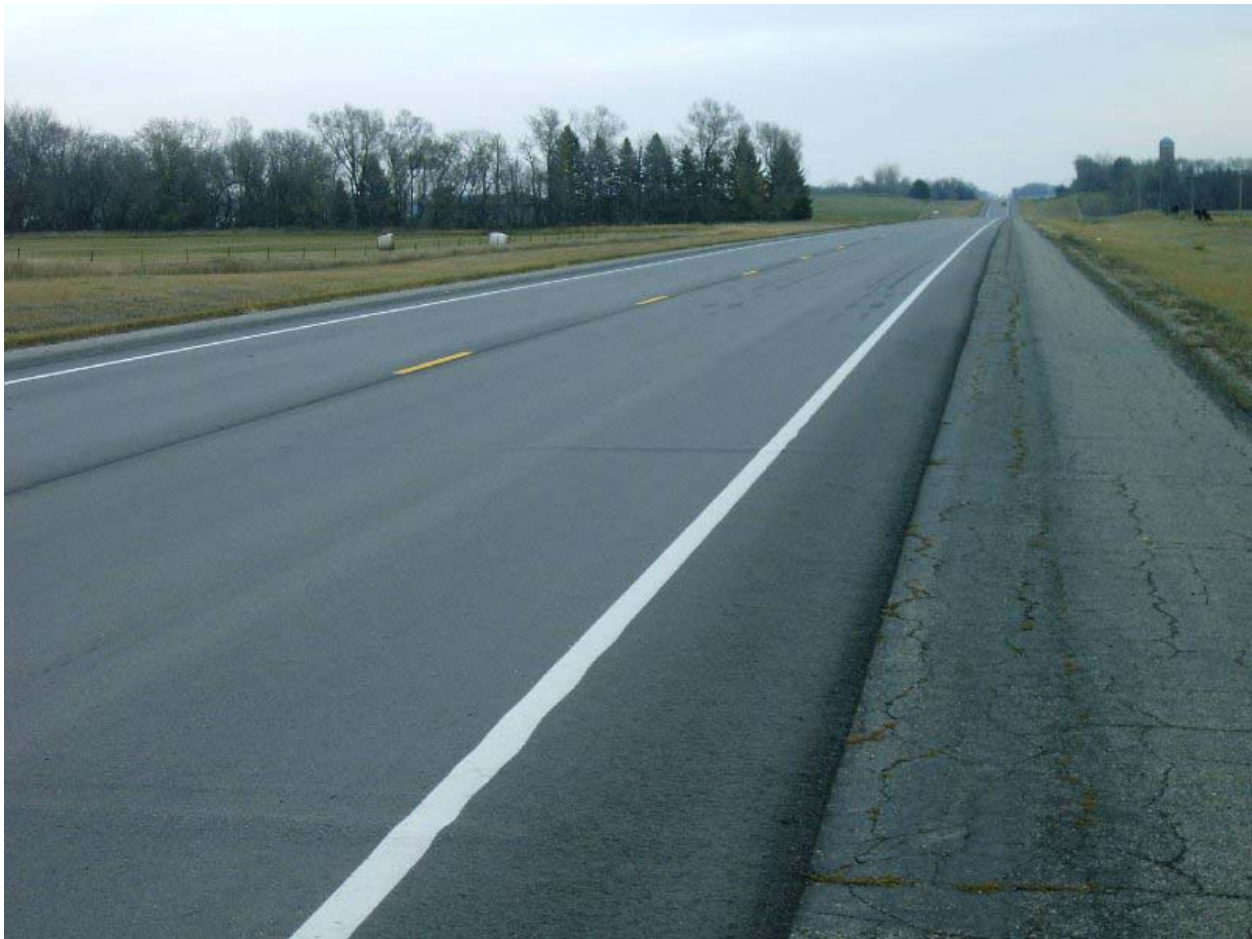
Figure 6.17. Bumps in overlay on US 212 in District 8.
