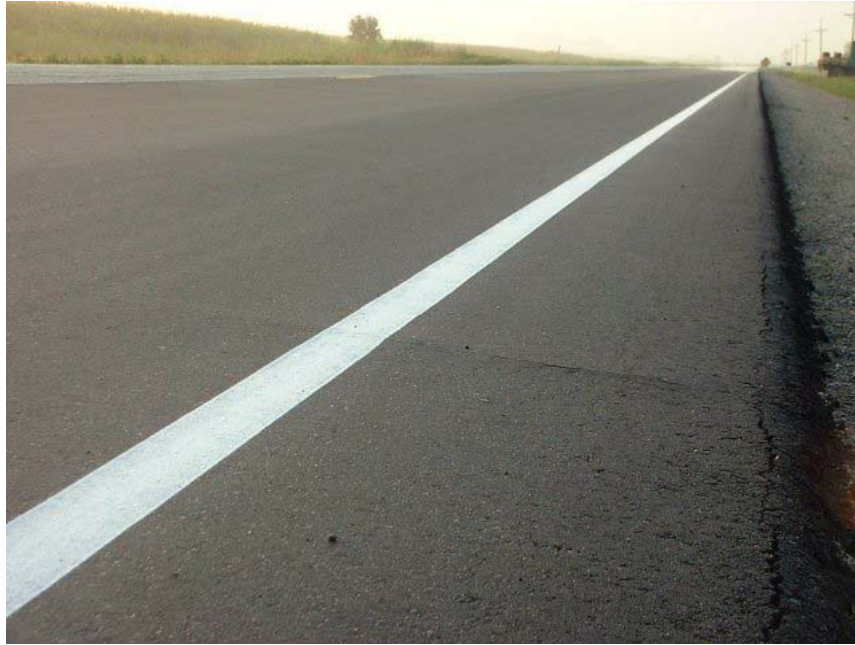
Figure 6.6. One of numerous small bumps found near milepost 34 on TH 22 near Mapleton, Minn.
