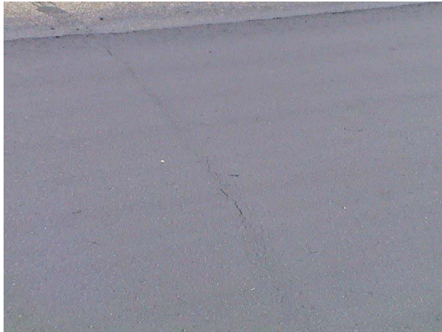
Figure 6.12. Bump at Sealed Crack at Lyon County CSAH 9.
