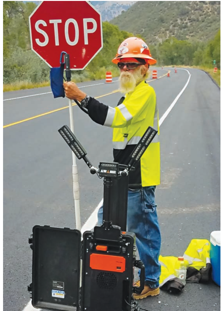
Flagger manning the AWARE System, on Highway 133 near Paonia, for United Companies.
