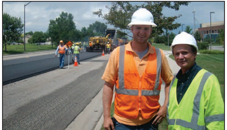
Tyler Newland, a recent CSU – CM graduate, shown left with Larry Schneider, City of Ft. Collins Streets Superintendent, is working as a Project Inspector for the city. He was involved in the paving work on both Horsetooth Rd. and S. Shields Road this summer.
