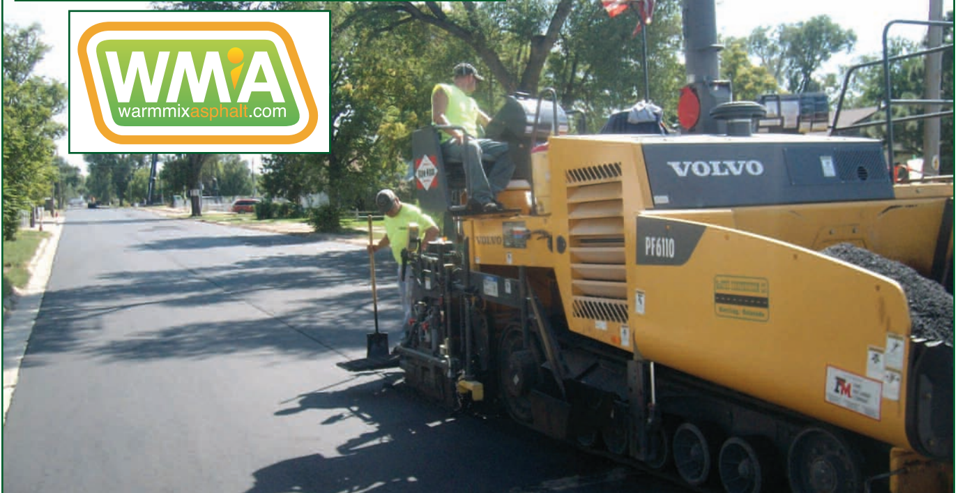
McAtee Construction placing warm mix asphalt on streets in the City of Sterling. All mixes contained 20% RAP.
