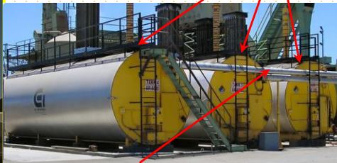
Storage Tank & Delivery Piping Heating System
